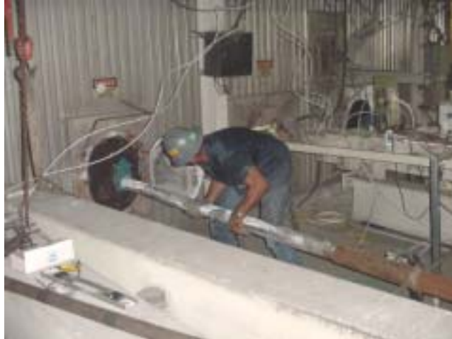
Figure 28. Photograph of Darren Garvis of Process Metrix assisting the insertion of the PPC probe into the Courtland recovery boiler.
