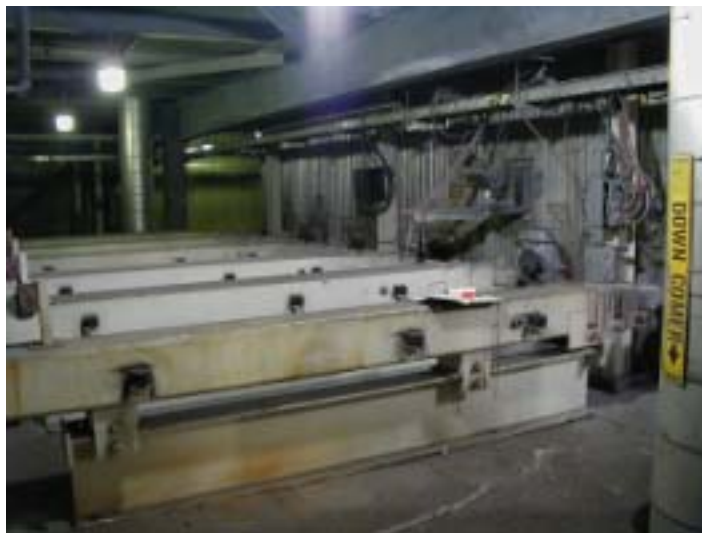
Figure 27. Photograph of six maintenance beams along the front wall of Courtland recovery boiler #3.
